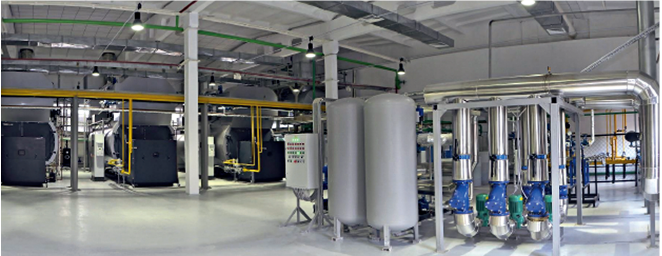
Energy centre with Vitomax boilers. These can already run on 100 percent hydrogen.
